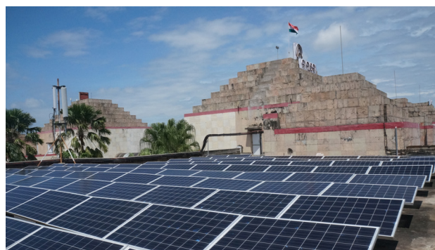
Roof-top solar panels - Corporate Office
