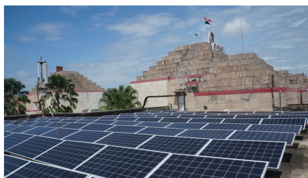
Roof-top solar panels - Corporate Office
