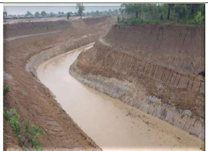
Nallah diversion along mine boundary
