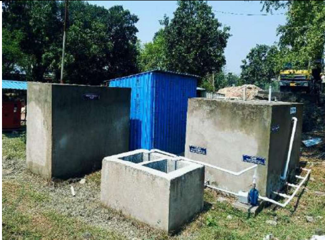
Effluent Treatment Plant
