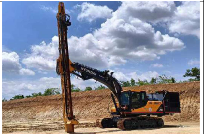
Drill Machine (Wet type)
